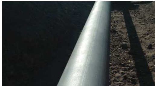
Pipe already cleaned to SP 10 (near white metal) and anchor profile of 2.5-5 mil.
