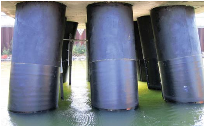
Shell Refinery - Deer Park, TX
